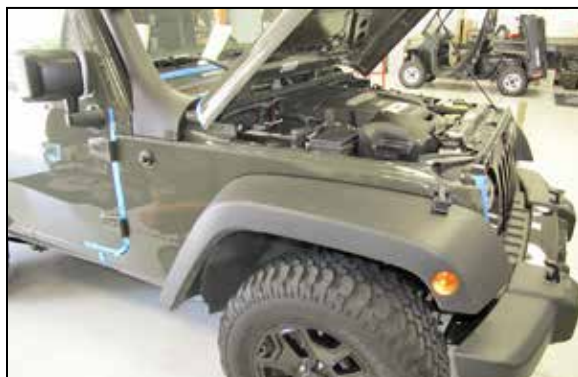
54. With an assistant, temporarily reinstall the fender onto the vehicle but do not secure it at this time. Adjust the snorkel for best fit and then secure the snorkel bracket to the inner cowl and the outer cowl to the snorkel with the factory hardware.
